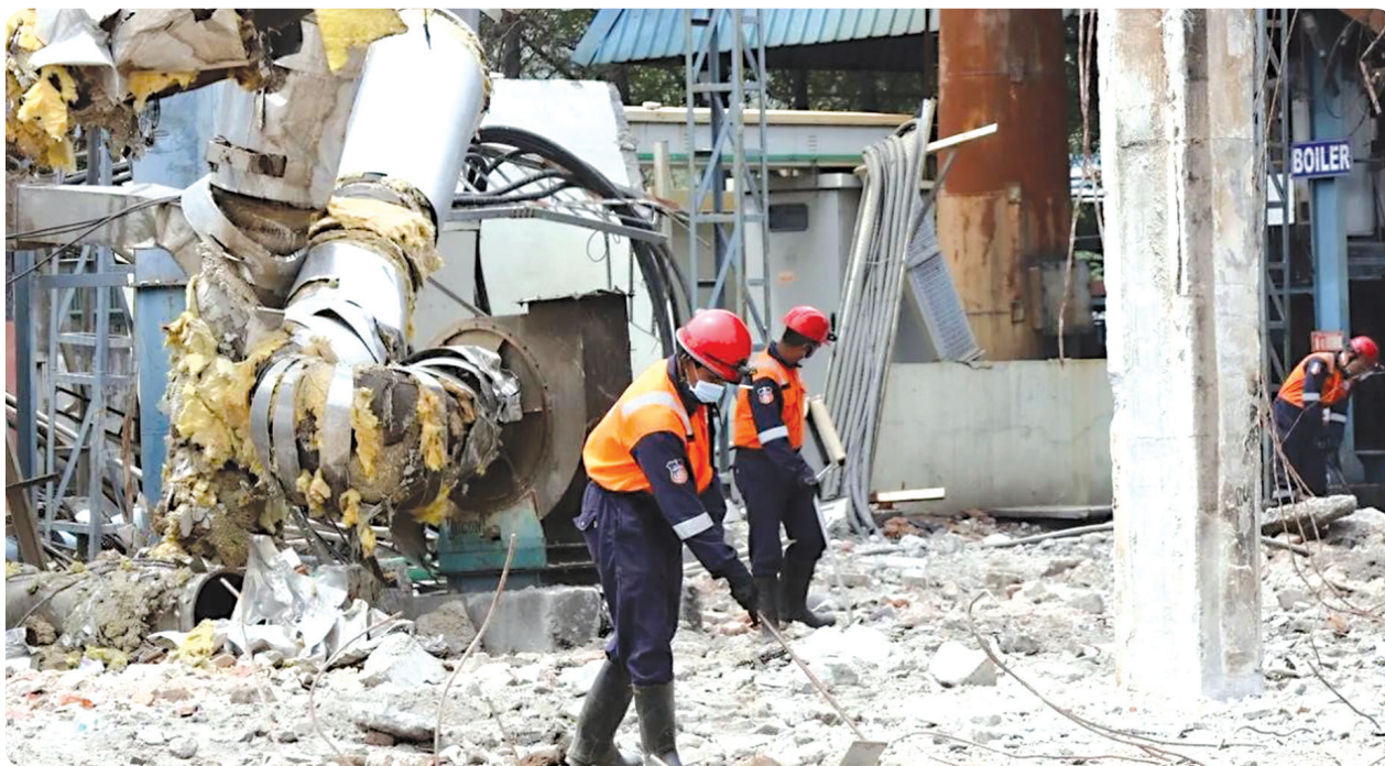
Figure 71: Personnel of NDRF, police and the fire department search for human remains at the blast site in Sigachi.
