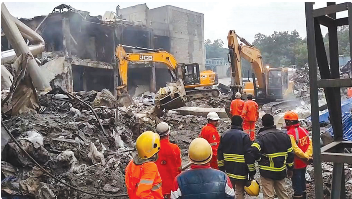
Figure 68: NDRF personnel conducting rescue operations at the explosion site.
