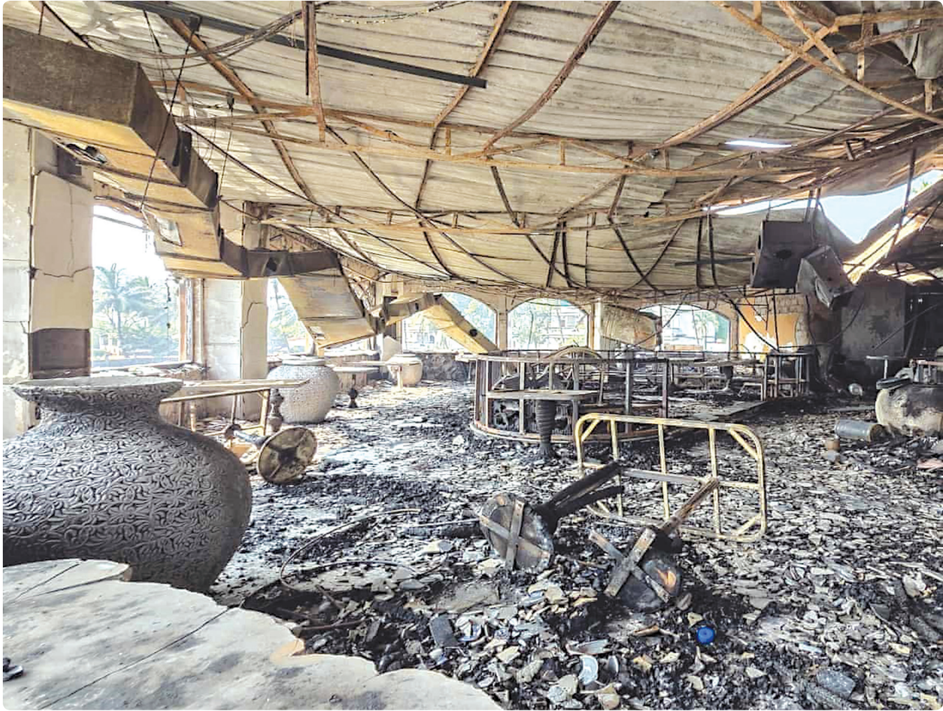
Figure 74: Aftermath of the Arpora nightclub fire showing structural damage.
